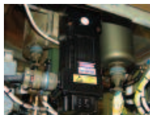
DC Motor Controller
